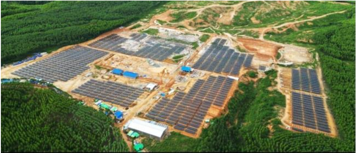
PV Solar 50Mw as renewable energy for Indonesia New Capital Nusantara Project
